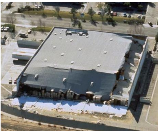
Figure 3. Photo of tilt-up building with the first bay of diaphragm caved in due to out-of-plane wall connection failure [source: EERI].
